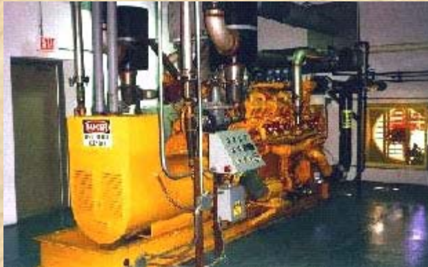
Internal Combustion Engine (range from 100 kW to 3 MW)
